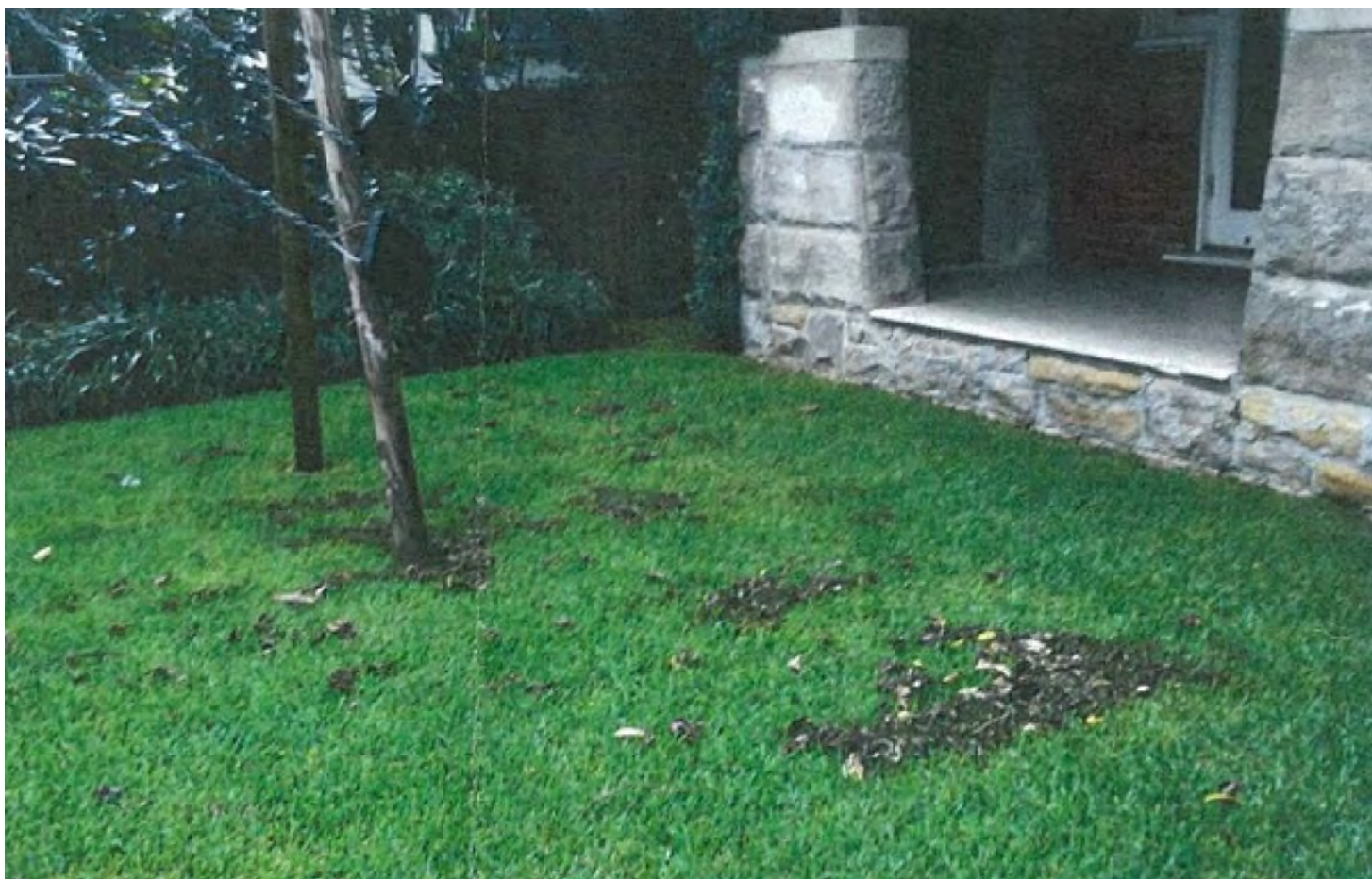
Lang Road, Centennial Park, showing settlement of leaves following flooding above height of raised front lawn.
